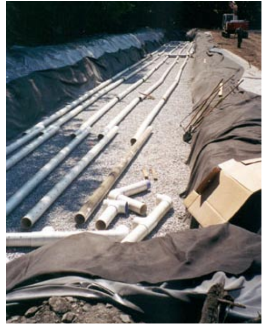
Passive Acid Mine Drainage Treatment System, Newkirk Tunnel
