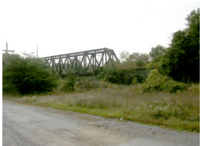
Figure 3. 11 The large steel through-truss bridge of the Bartram Trail provides the opportunity for an interpretative point with great views of the Kernsville Dam and river.
